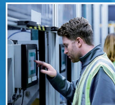
Factory control panels
